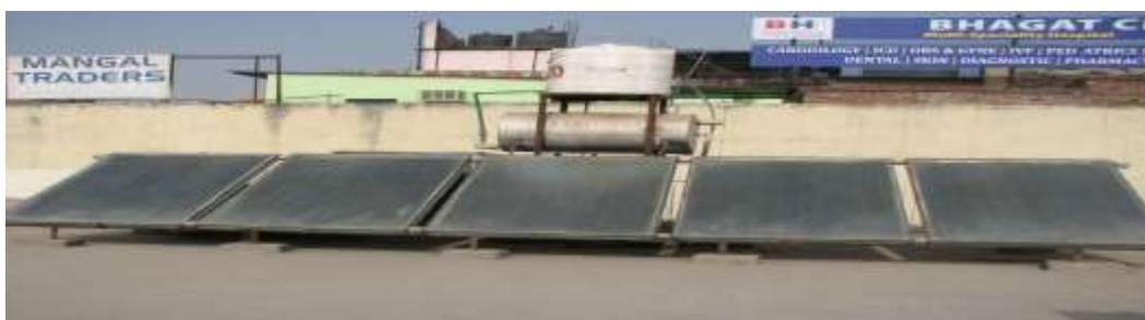
Figure 2: Solar panels used for water heating
