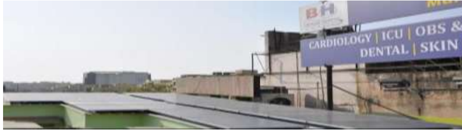
Figure 1: Installed Solar Panel located at the hospital
